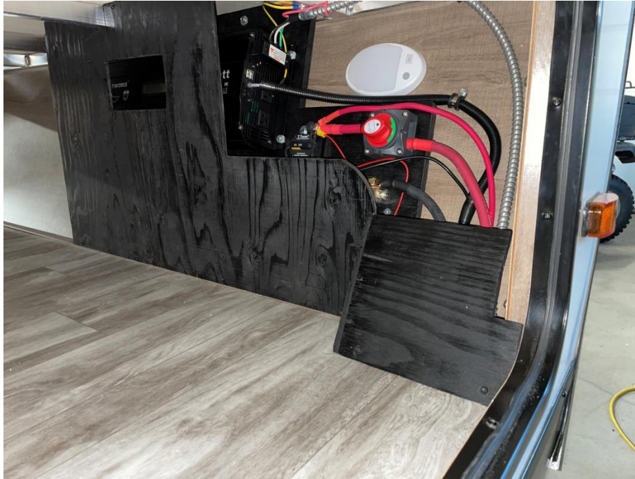
Inverter module in place with protective panels
