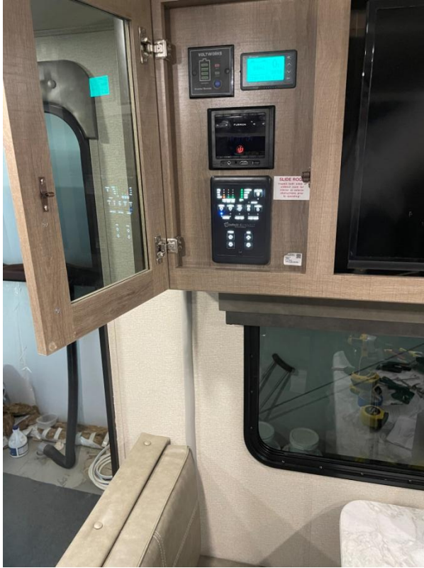
Inverter control panel and battery monitor in cabinet
