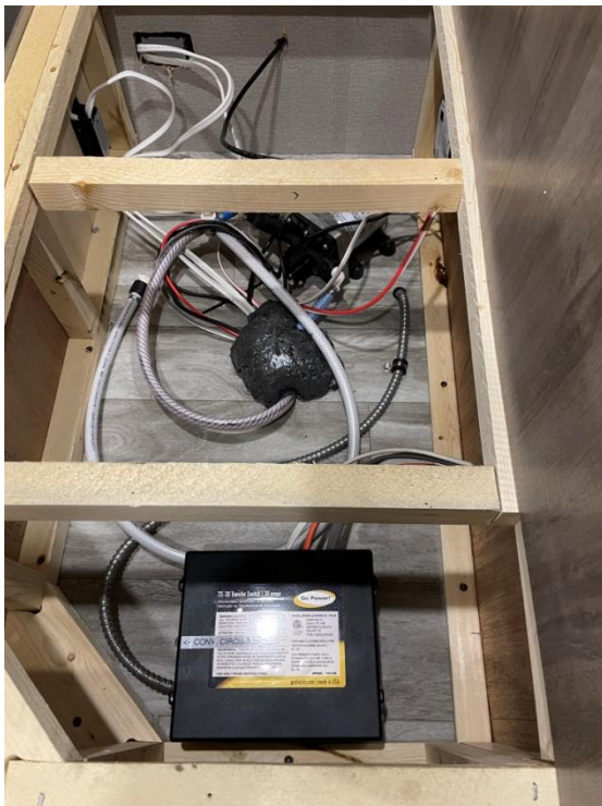
ATS mounting location under aft dinette bench
