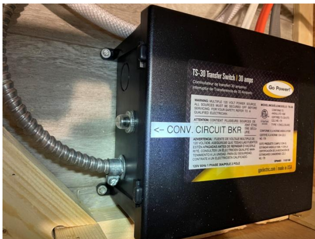
Location of the new 15A/120V push button circuit breaker
