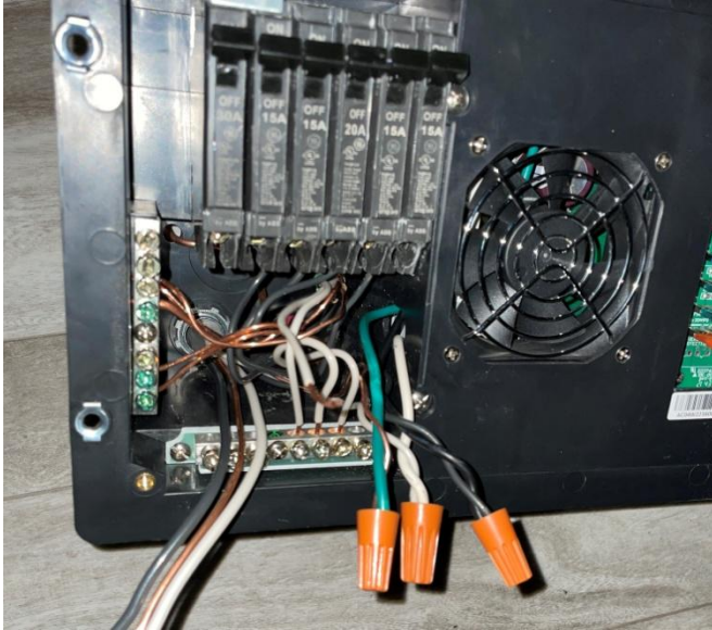
Converter section power wires connected to 14/2 NM cable
