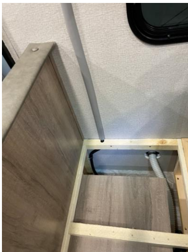
Wiremold is flush with top of stringer
