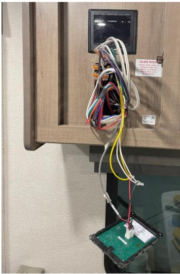
Wiring behind lower control panel
